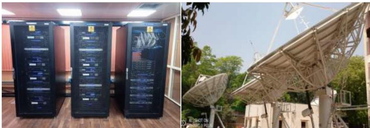
Figure 5: High-end servers and antenna of the MMDRPS at IMD, New Delhi.
